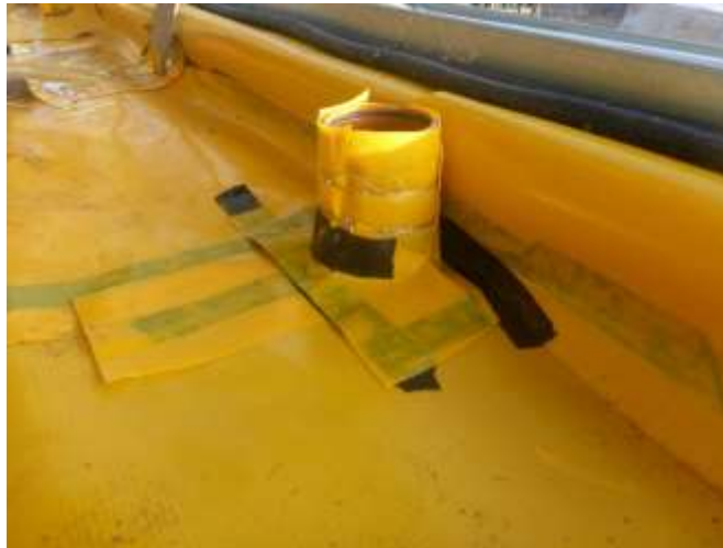
Plate 4: Gas membrane taken up 150mm and sealed with double sided tape around service penetration
