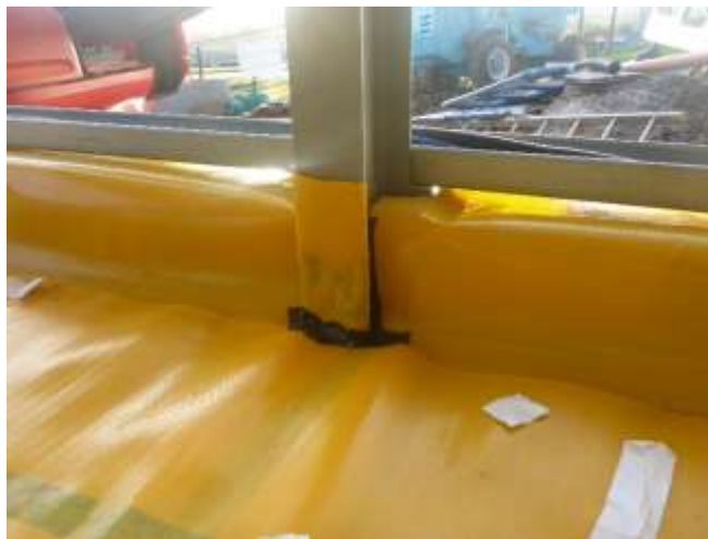
Plate 5: Gas membrane taken up 150mm and sealed with double sided tape around stanchions
